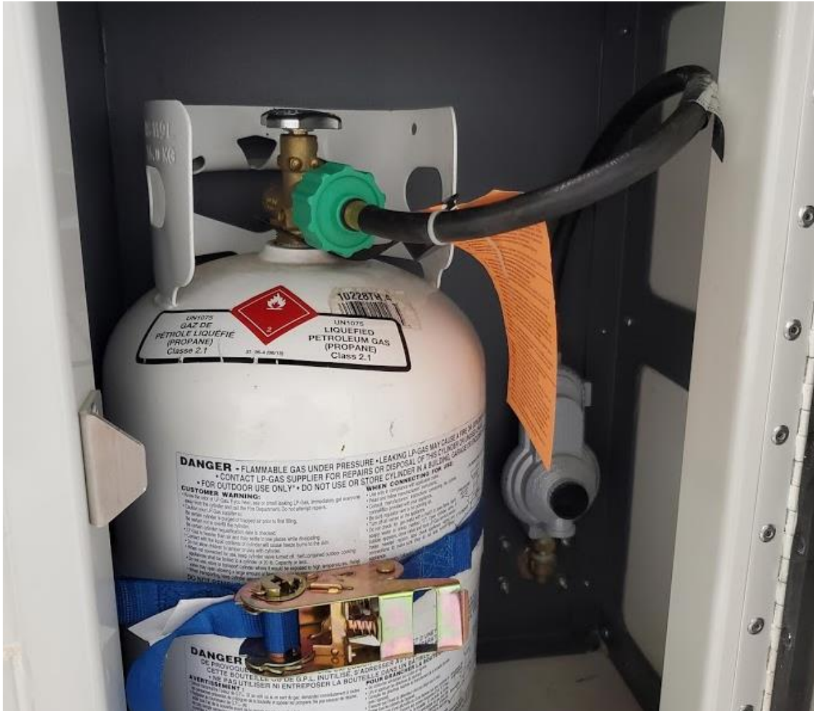
Propane tank in cabinet with ratchet strap.
