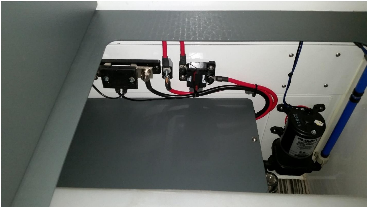
Battery box, water tank, water pump, tank drain, strainer, DC main resettable breaker, located under front dinette seat
